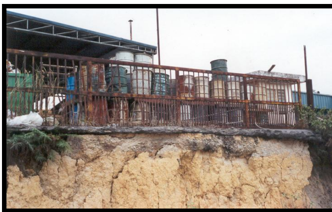
Figure 1: Example of improper storage of schedule wastes at the edge of slope
