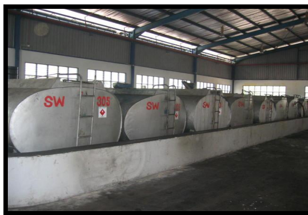
Figure 4: Storage tanks for waste oil. The capacity of the containment should be 110% of the largest container stored.
